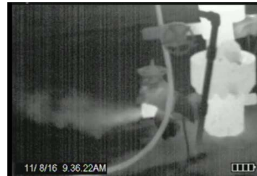
Leak from a wellhead
