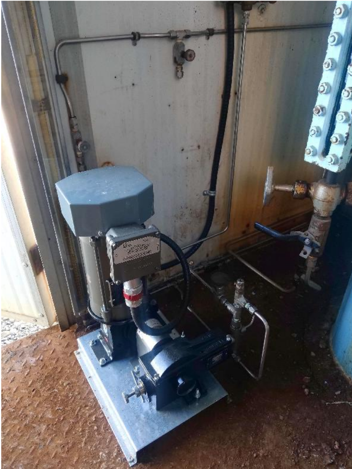
Figure 1: Olds 02-02-031-02 W5 MCP – Standard Electric Final Install (Simplex)
