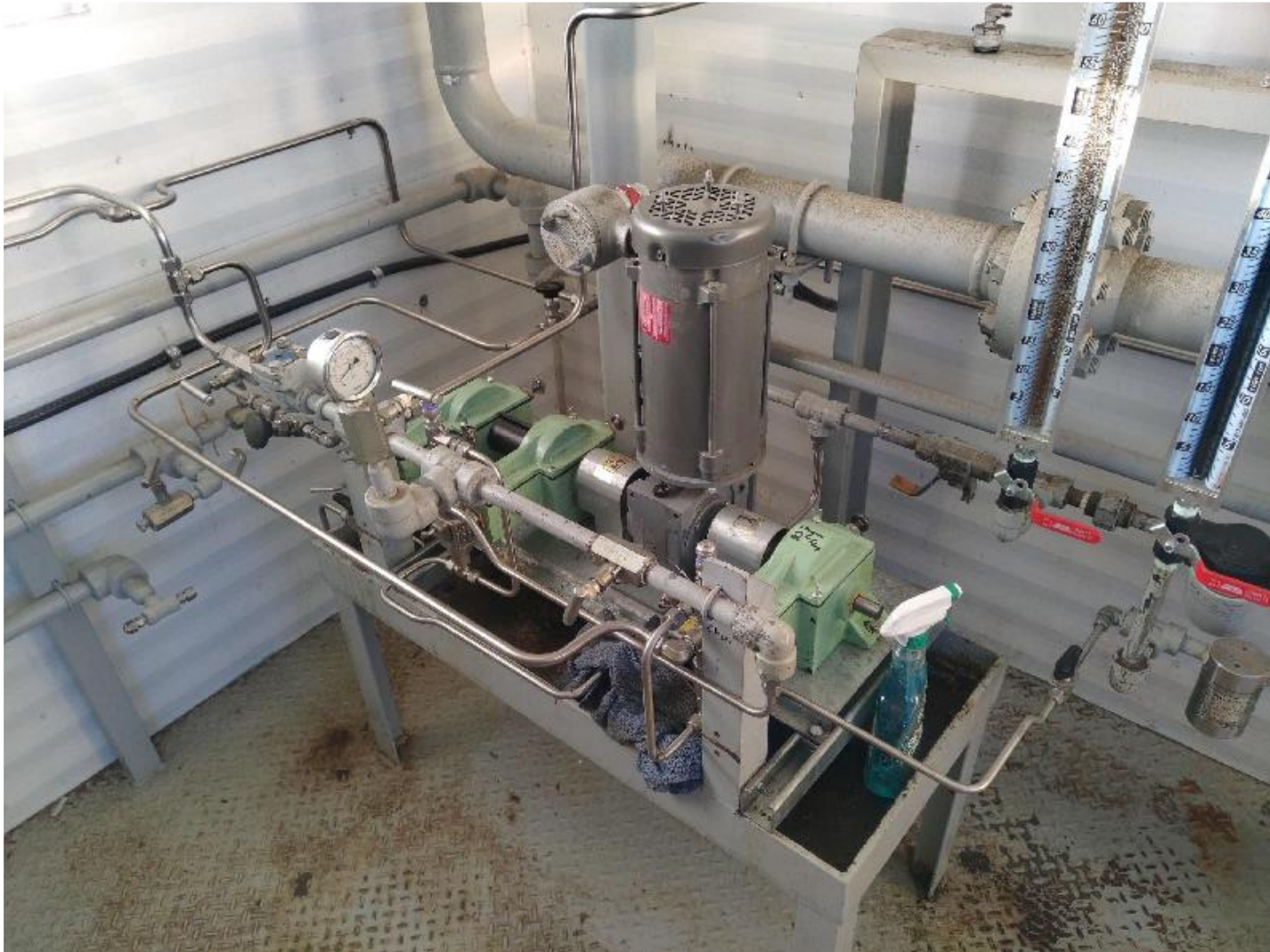
Figure 3: Olds 07-02-030-01 W5 MCP– Standard Electric Final Install (Triplex)
