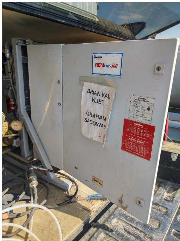
Picture 3. Photo of the Emeas Skid flow computer which was used to measure the vent rate of pre and post plunger head retrofits.
