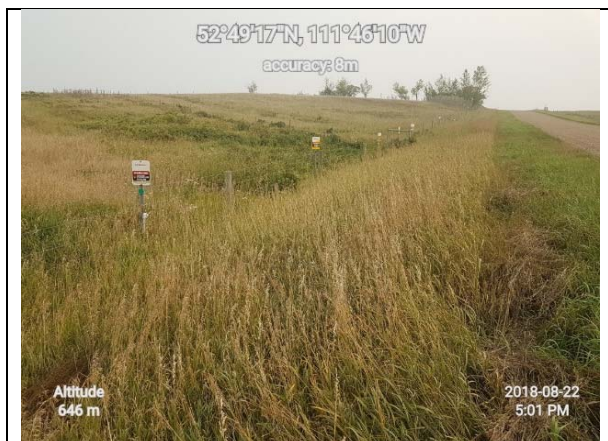
Plate D-9. View south along the abandoned pipeline segment near KP 136.7 at NE 26-44-13 W4M, where the removed segment begins.
