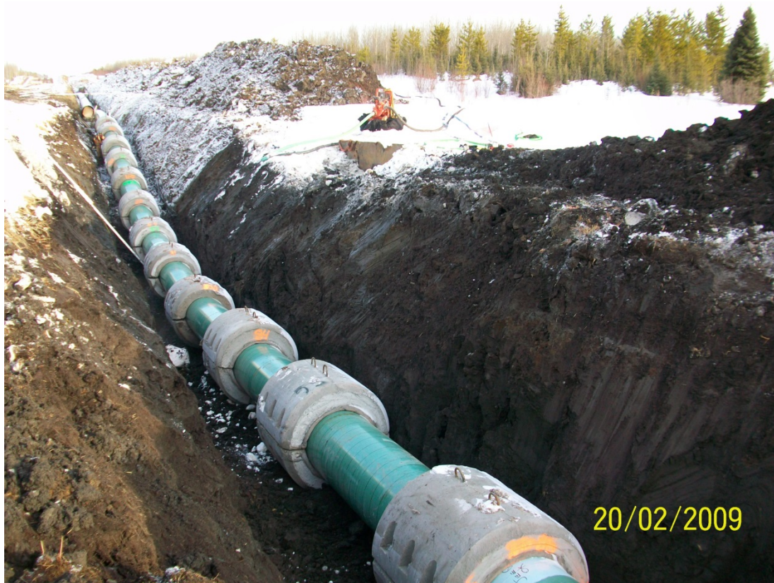
Figure 2 Concrete River (bolt-on) Weight (photo courtesy of J. Harris)
