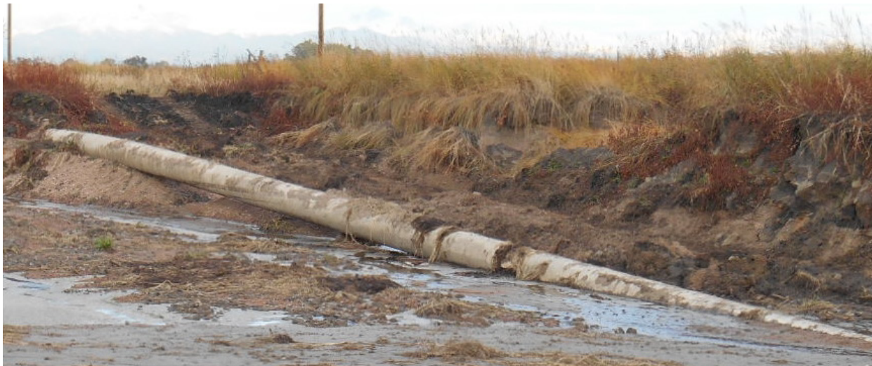
Figure 18 Exposed Continuous Concrete Coating, no Noticeable Deterioration after Approximately 8 Years (photo courtesy of G. Connors, PipeSak®)
