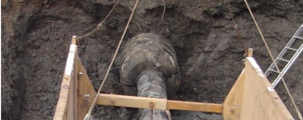
Figure 17 Concrete Bolt-on Weight, Approximately 60 Years Old, with no Noticeable Deterioration and the Weight Halves Still Locked Together (photo courtesy of D. Madden, TransCanada Pipelines)
