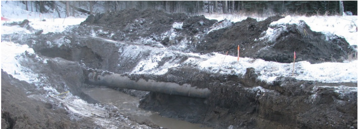
Figure 20 Soil and Water Conditions in Area of Excavated Screw Anchor in Northeast BC (photo courtesy of A. Brown, AHB Consulting)
