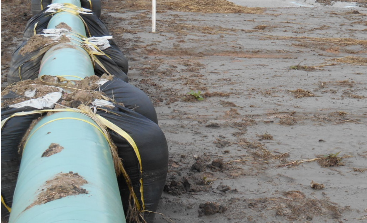
Figure 22 Exposed Geotextile Bag Weights, no Noticeable Deterioration of Tears. Weights Were Approximately 8 Years Old (photo courtesy of G. Connors, PipeSak®)
