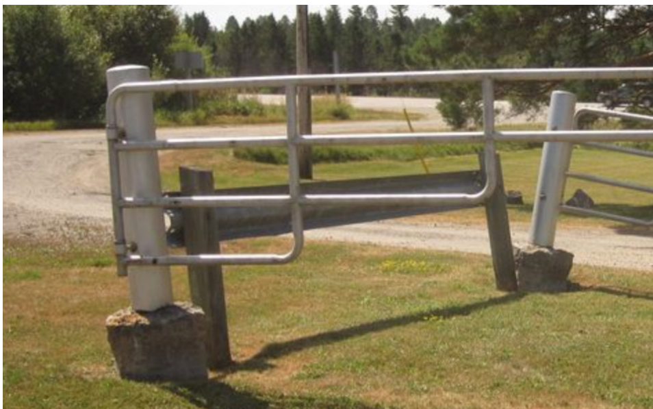
Figure 29 Frost Jacking of Posts (Woodgears, 2018)
