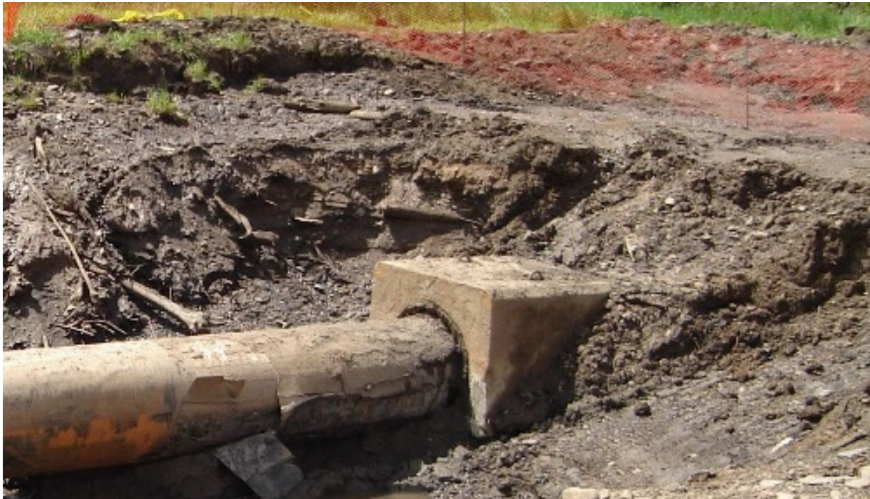
Figure 15 Concrete Set-on Weight, Over 50 Years Old, with no Noticeable Deterioration (photo courtesy of D. Madden, TransCanada Pipelines)
