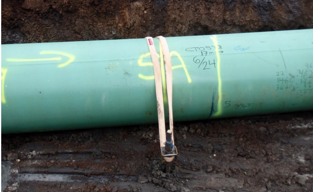
Figure 9 Example (1) Steel Screw Anchor and Polyester Strap Saddle and Connection (photo courtesy of A. Brown, AHB Consulting)
