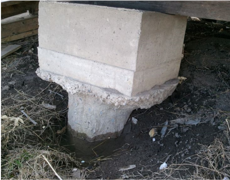
Figure 28 Frost Jacking of a Concrete Footing Foundation (Woodgears, 2018)
