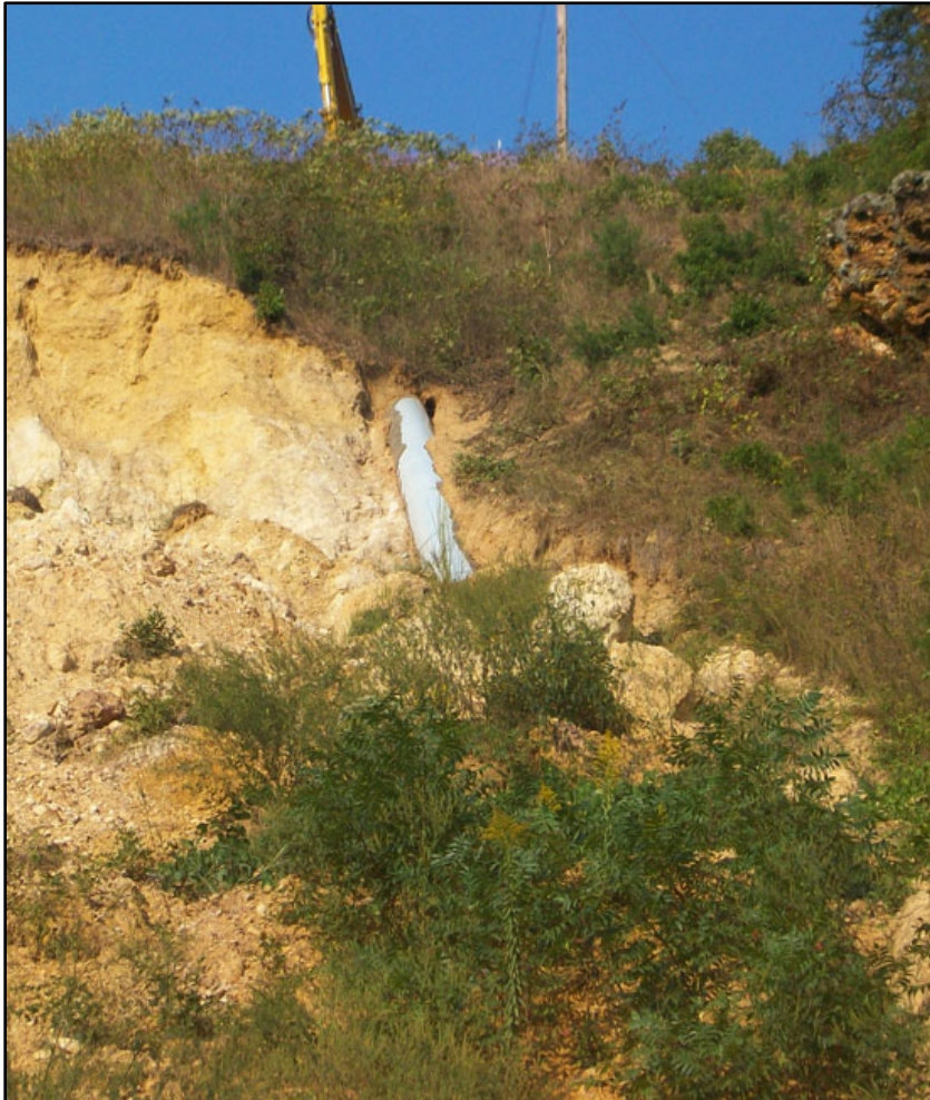
Figure G-1. Pipeline exposure caused by mass movement of soil on steep terrain. (source: Jones Contractors, Inc., 2014).
