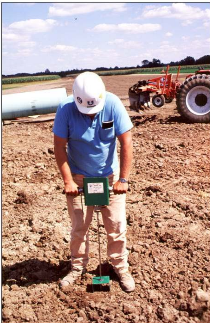
Figure N-7. Environmental inspector (pipelines) conducting soil cone penetrometer testing to verify the efficacy of deep-ripping (sub-soiling) operations in the trench and workspace areas of a pipeline ROW (photo: R.A. McBride).
