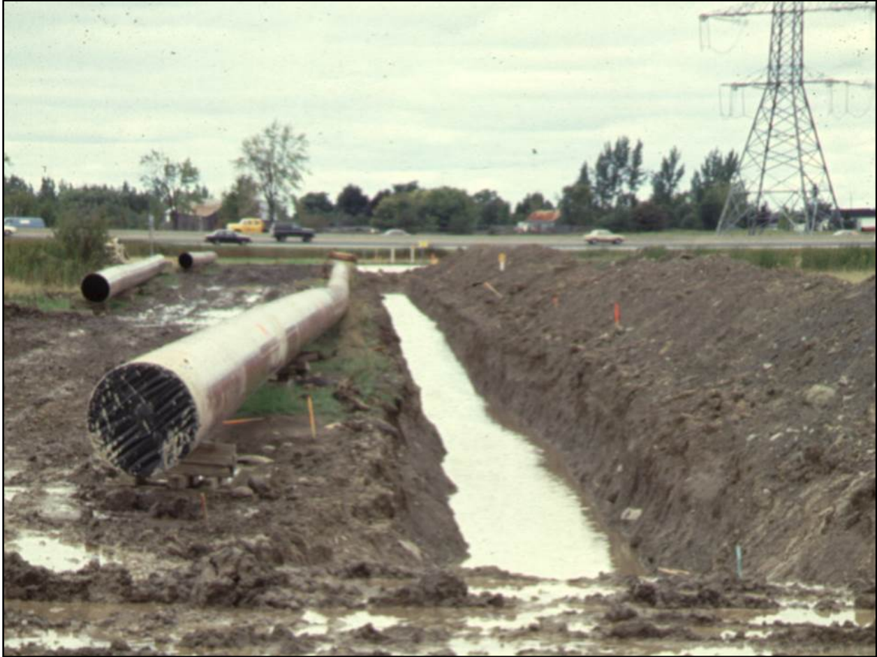
Figure Q-2. Inundation of an open pipeline trench near Milton, ON after an extended period of heavy, sustained rainfall and surface runoff (photo: R.A. McBride).
