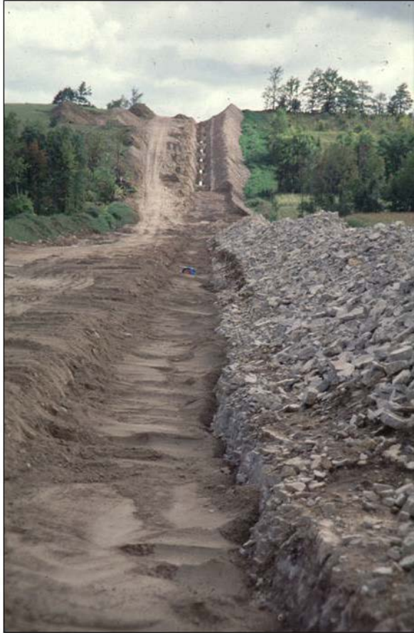
Figure N-2. Back-filling of pipeline trench in variable terrain ( foreground - shallow to bedrock; background - steep topography over drumlin) (photo: R.A. McBride).
