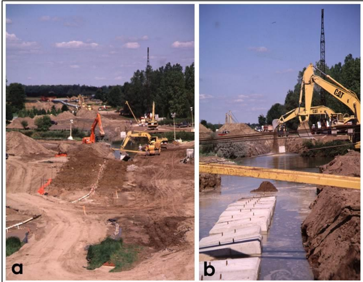
Figure 2.3: Installation of a natural gas pipeline a) across the Nith River near Ayr, ON, with b) concrete pipe weights reducing exposure risk from buoyancy (photos: R.A. McBride).
