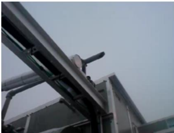
Figure 7 - GasPro PRV-900 Discharge
