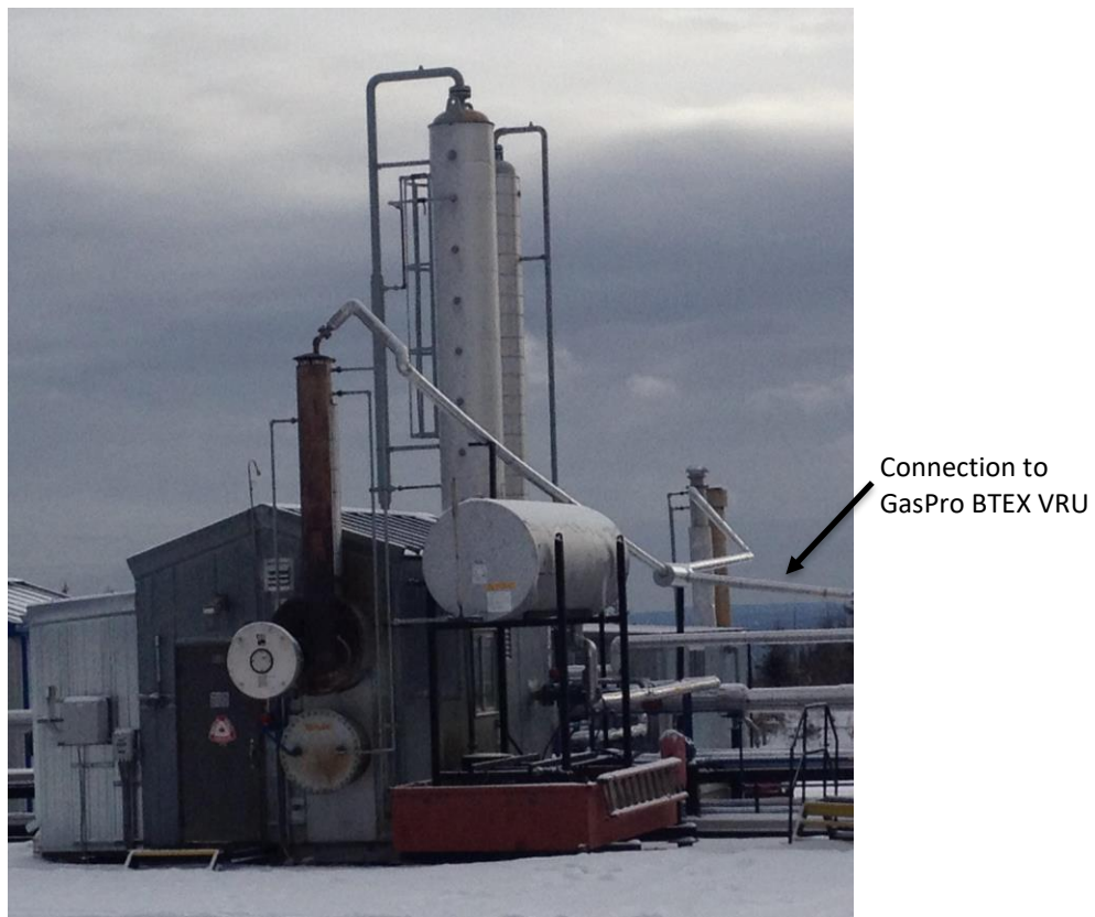
Figure 3 - Two Dehydration Units with Still Overheads Piped to GasPro BTEX VRU
