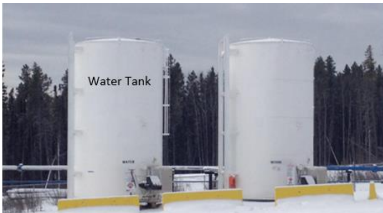
Figure 6 - Methanol and Produced Water Storage Tanks
