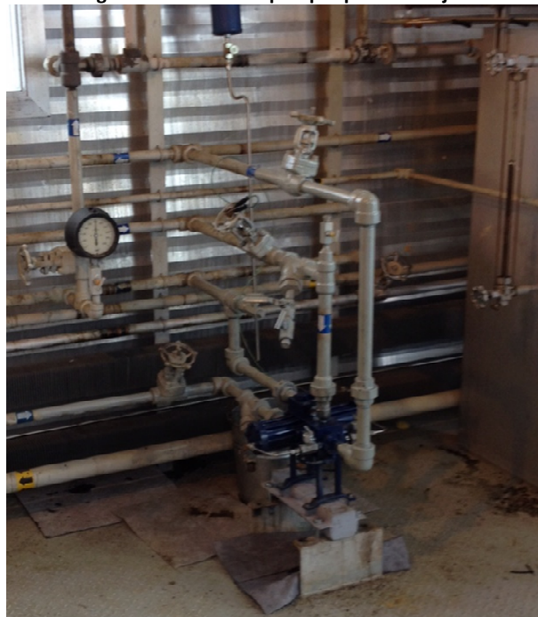
Figure 5: Kimray 1720PV pump as installed in Hanna 4-29
