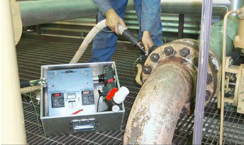
Figure 5: The Hi-Flow sampler being used to measure a flange leak rate.
