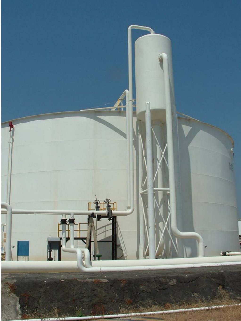
Figure 4: A photograph of a typical vapour recovery tower elevated above the storage tank.
