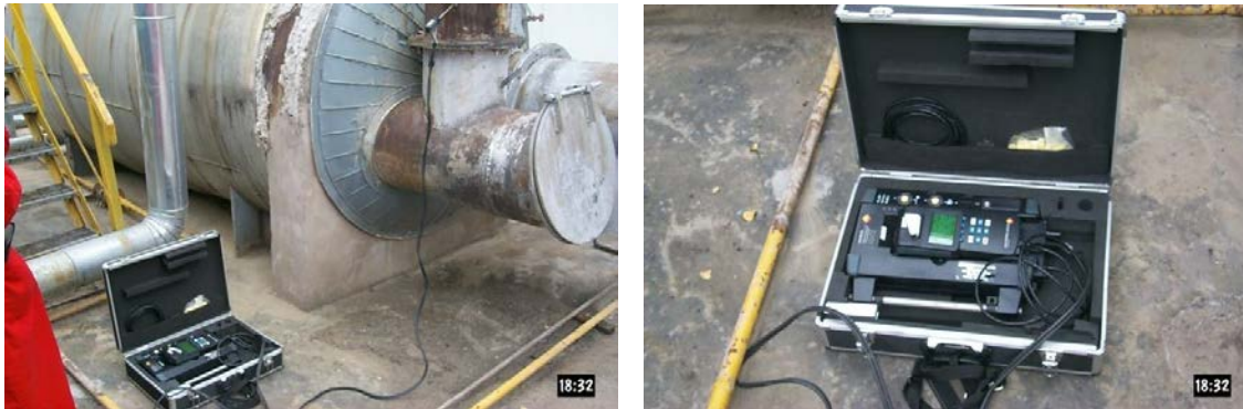
Figure 8: Photographs of combustion test being conducted using a portable combustion analyzer.
