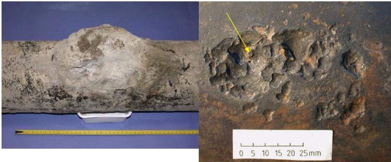
Figure 1. Leak site on underground natural gas transmission pipeline (attributed to AC corrosion) before and after cleaning. The arrow indicates the leak. [7]
