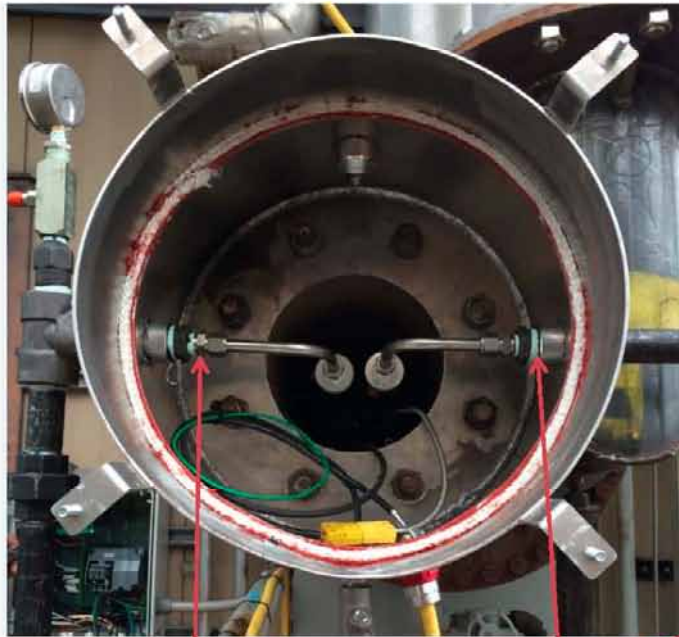
High Pressure Piping to Main Burner
