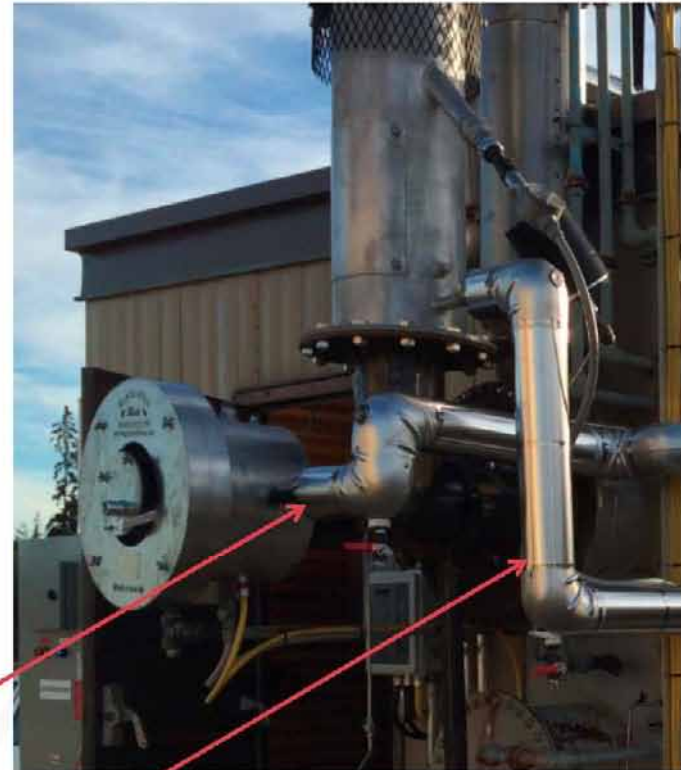
Low Pressure Piping to Aux Burner
