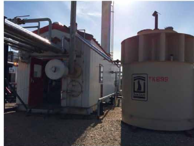
Tank Safe Exists
