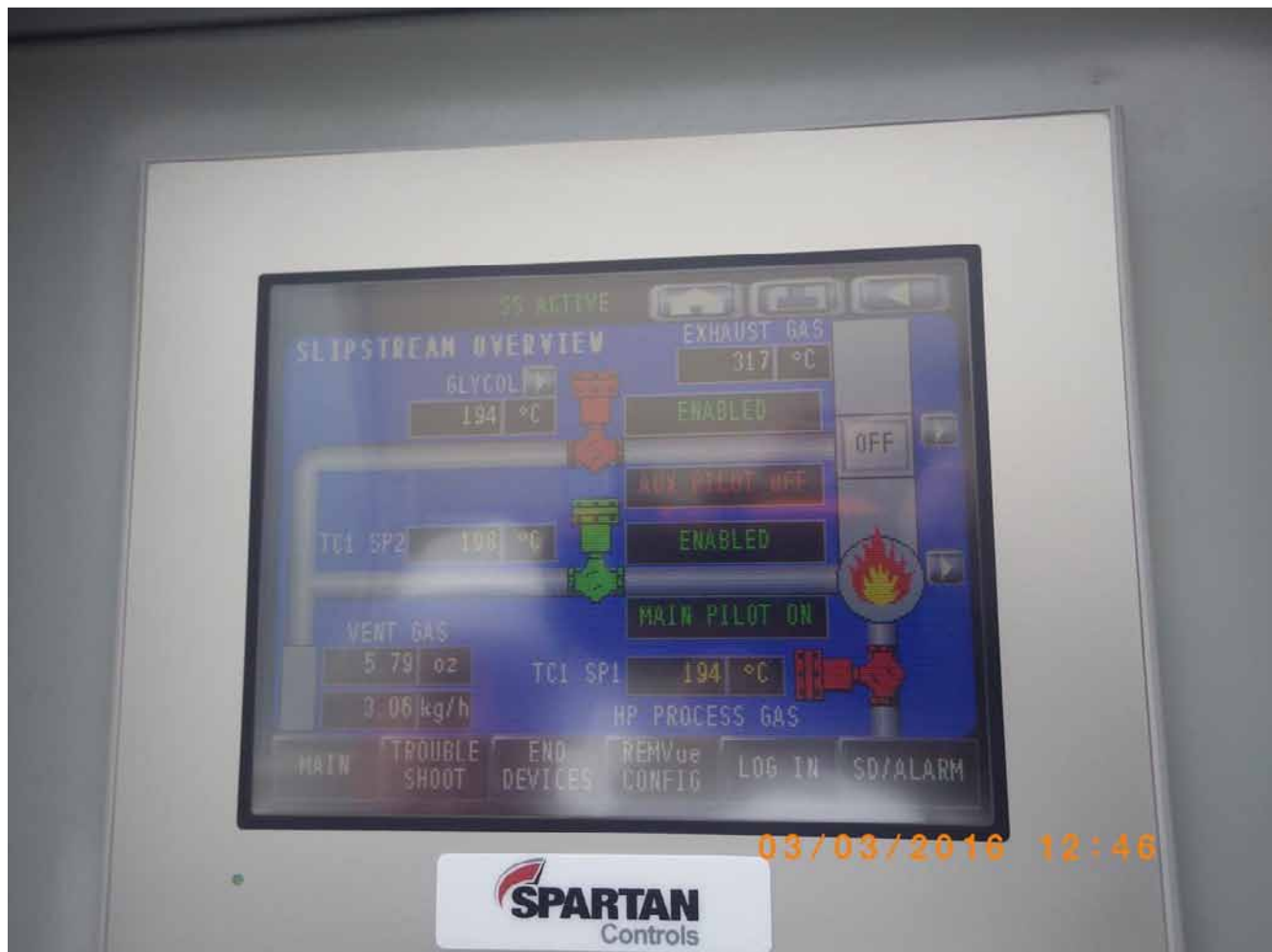
Photo 1: Spartan Control Panel showing Main Burner Running (green colored valve)
