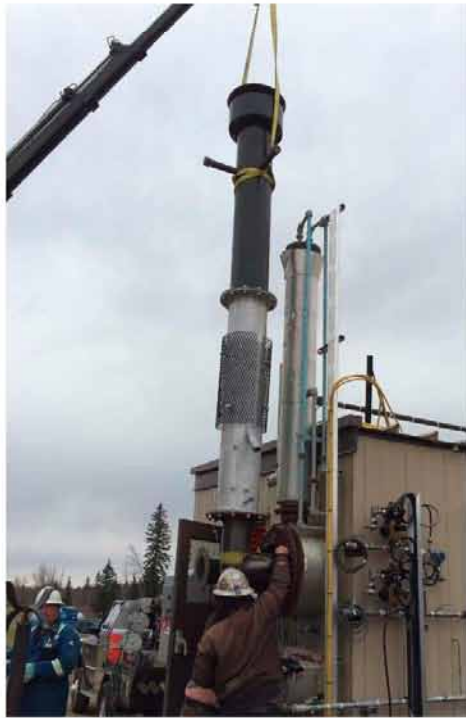
12" Aux Burner and Stack
