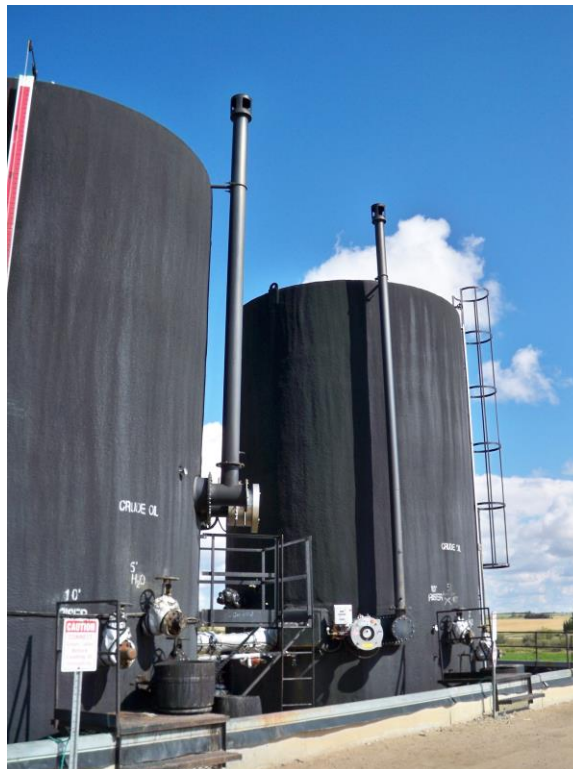
Figure 8: CHOPS Storage Tanks and Burners
