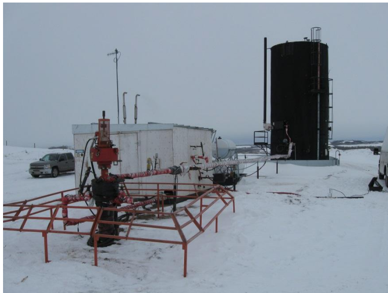
Figure 2: Typical CHOPS Site Installation
